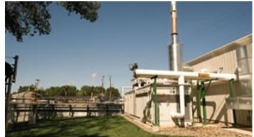
Gundersen Lutheran and City Brewery in La Crosse, Wis., powered up a first-of-its-kind combined heat and power project in 2009. The renewable energy project generates three million kW hours per year by using waste biogas discharged from the City Brewery waste treatment process and turning it into electricity.
